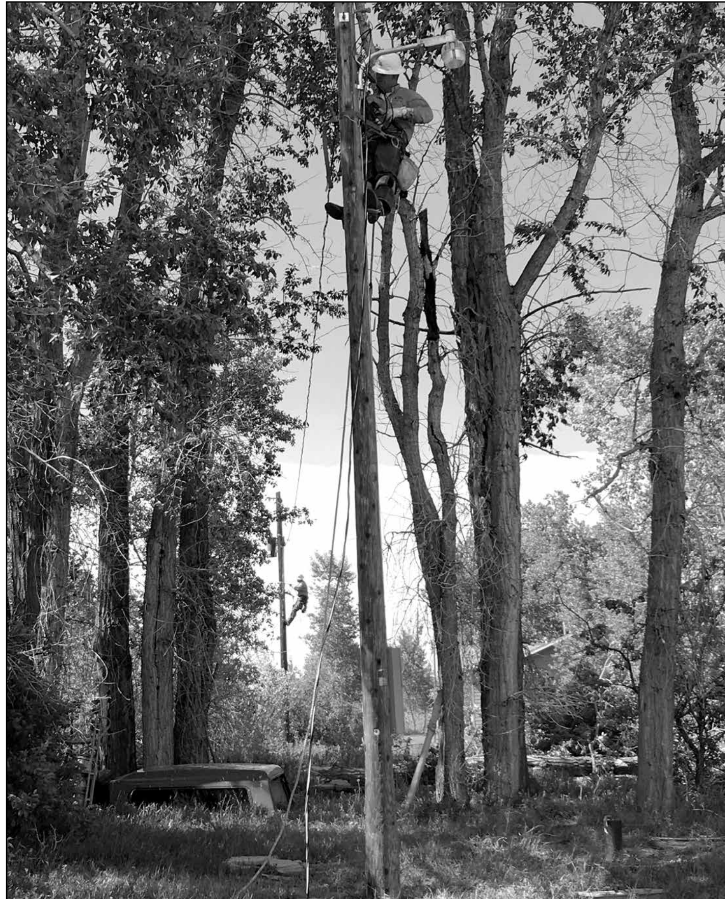
Jesse Lohmiller (foreground) and Eric McDonald replace service conductor that was torn down by a falling tree.
