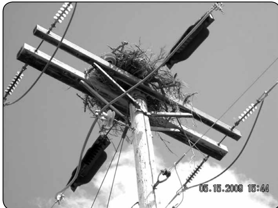
Above: Active-incomplete Osprey nest on a raptor-safe pole. It's easy to see how this can become a problem!
